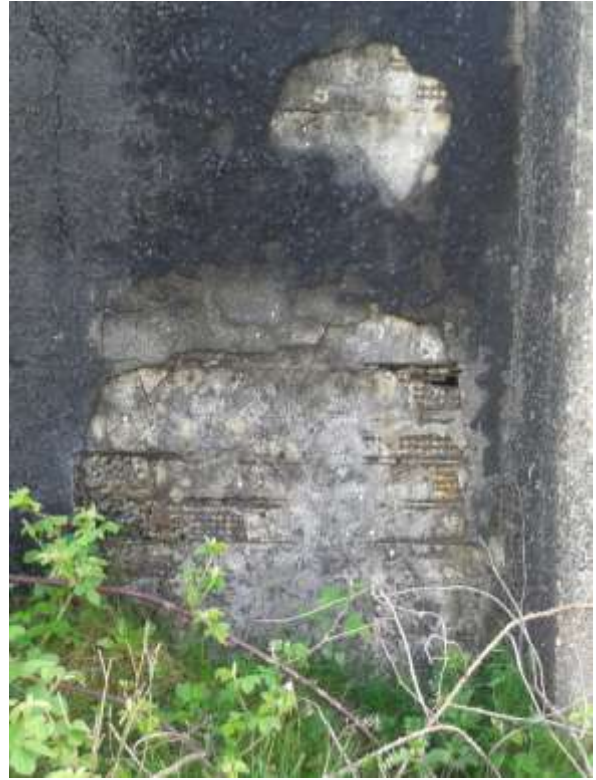
Photograph 8 - Spalled concrete / exposed reinforcement - 31/05/2019
