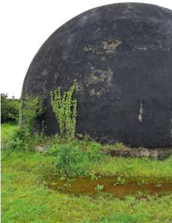
Photograph 9 - Vegetative growth to dome - 31/05/2019
