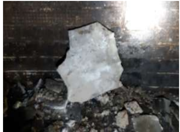
Photograph 12 - Concrete debris fallen from structure - 31/05/2019
