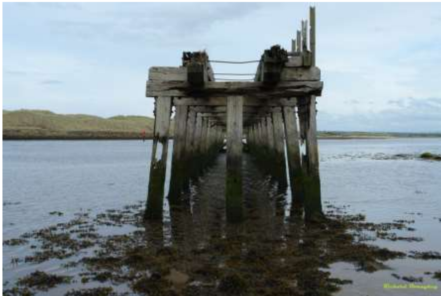
5 Industrial Heritage – remains of 19 th Century Railway Viaduct, built to assist in construction of the Barmouth Navigation Scheme
