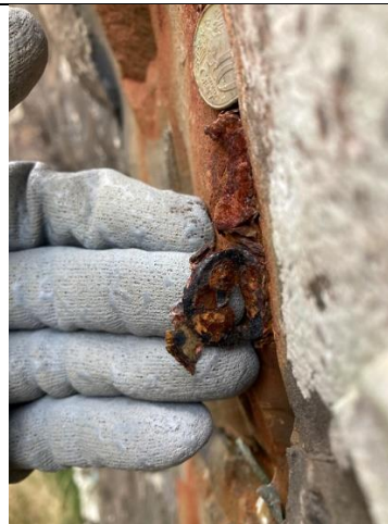
Figure 2 – Area 1 – Detail showing the condition of the coins in this area.
